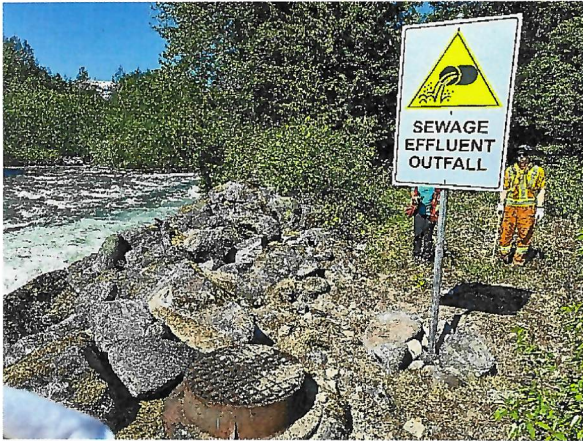
Photo 1: WWTP outfall signage located above outfall and adjacent to manhole access river right of Cheakamus River, May 15, 2023.
