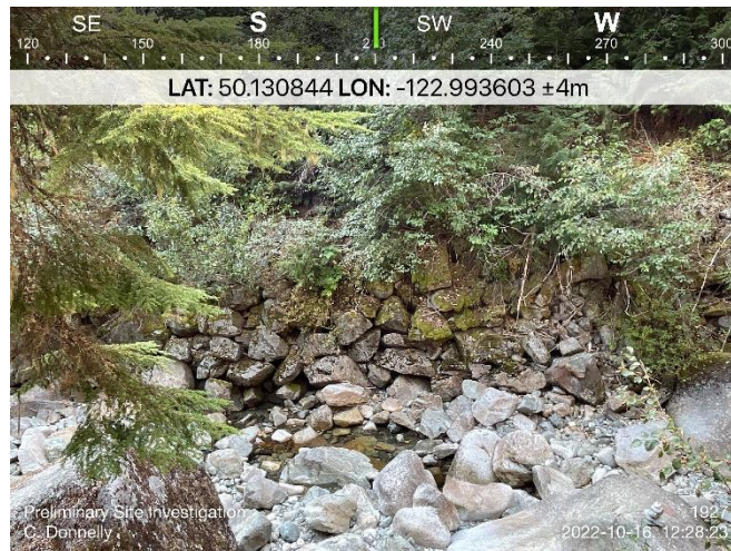
Figure 2: South of the existing bridge on the southwest bank, the slope is covered in large angular rocks.
