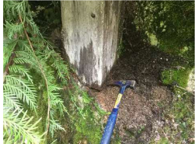
Photo 14 North approach boardwalk post condition
