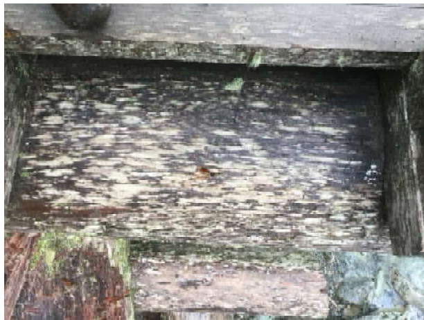
Photo 15 Upstream stringer condition
