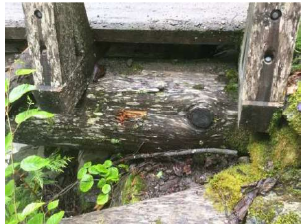
Photo 16 Downstream stringer condition
