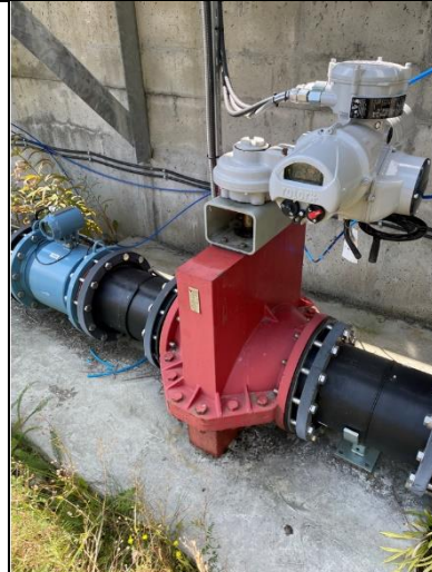
Outdoor control valve without any heat tracing or insulation.
