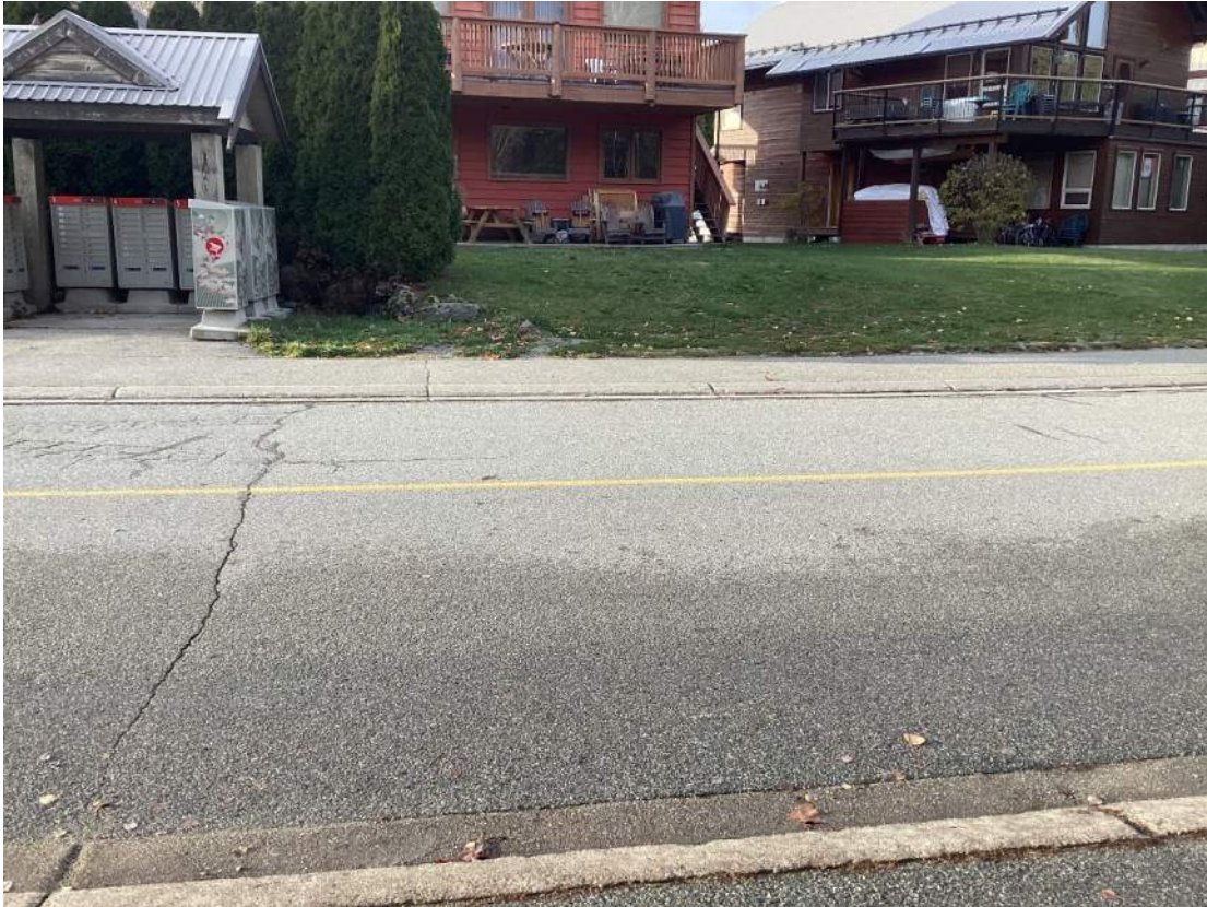
Photo S2-16.1: Cluster S2-16 General Location Looking Northwest Towards 7307 Spruce Grove Way
