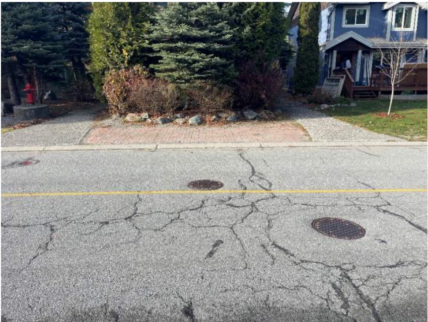
Photo W4-22.1: Cluster W4-22 General Location Looking Northwest Towards 7277/7281 Spruce Grove Way Approximately 1.2m from edge of curb in road (from GPR)
