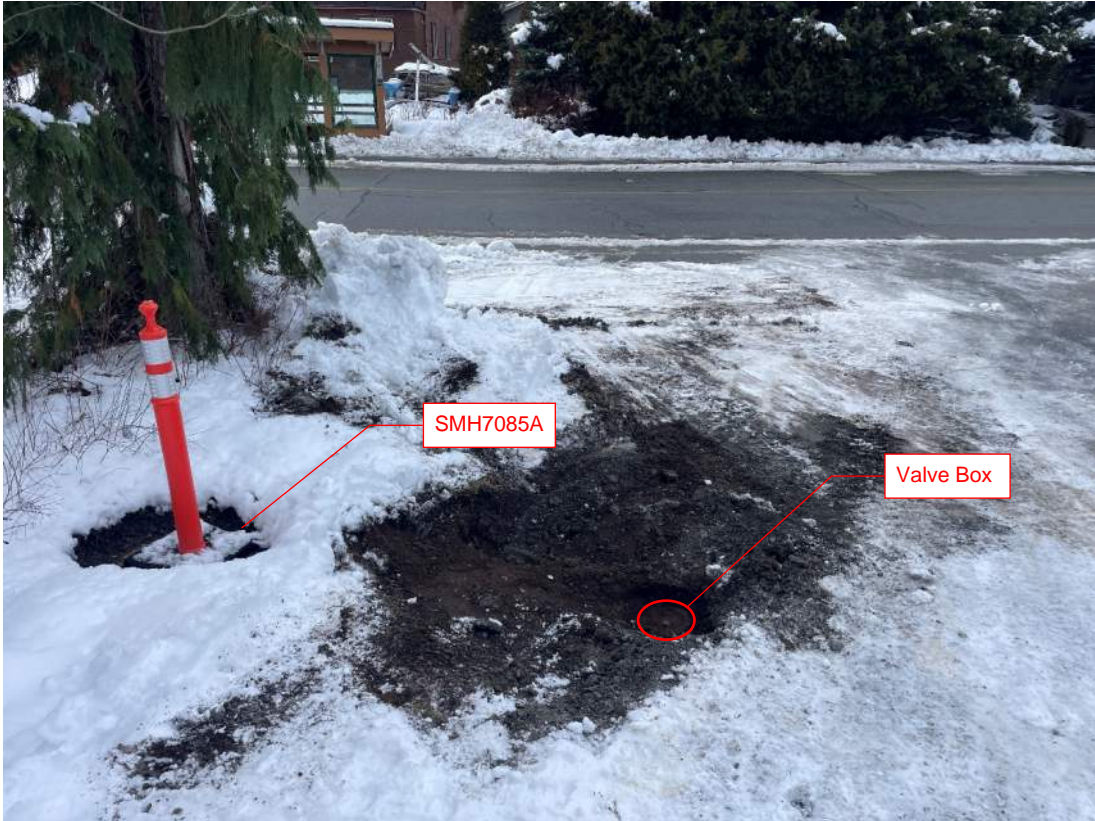
Photo S2-19.1: Cluster S2-19 General Location Looking Towards Spruce Grove Way at S126 Sewer Lift Station
