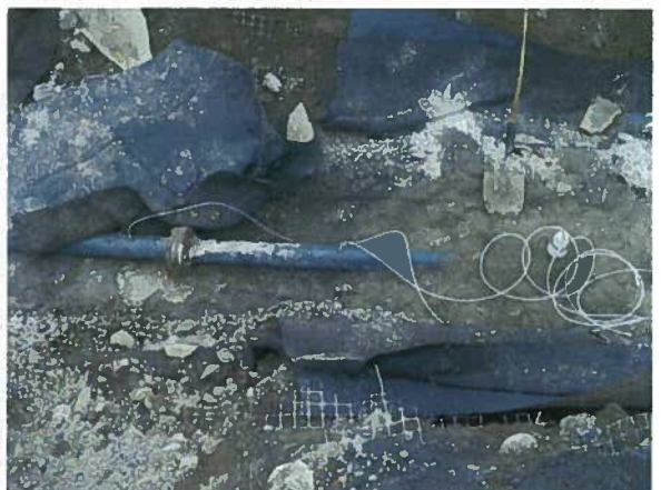
Photograph 6: Sampling Tubes near Orifice Plate (May 10, 2011)
