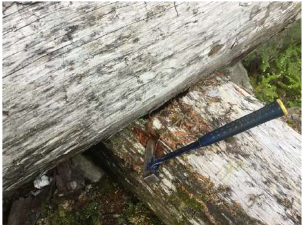
Photo 10 Typical sill condition
