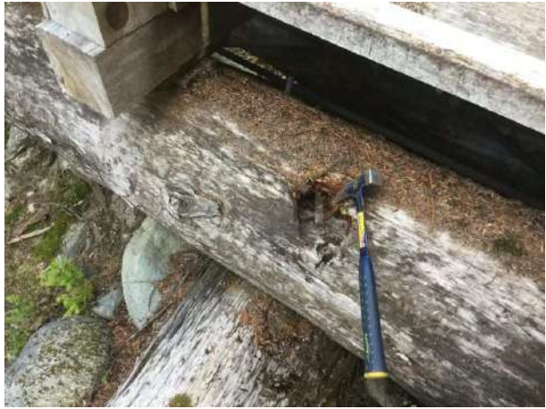
Photo 12 Typical decay in stringer
