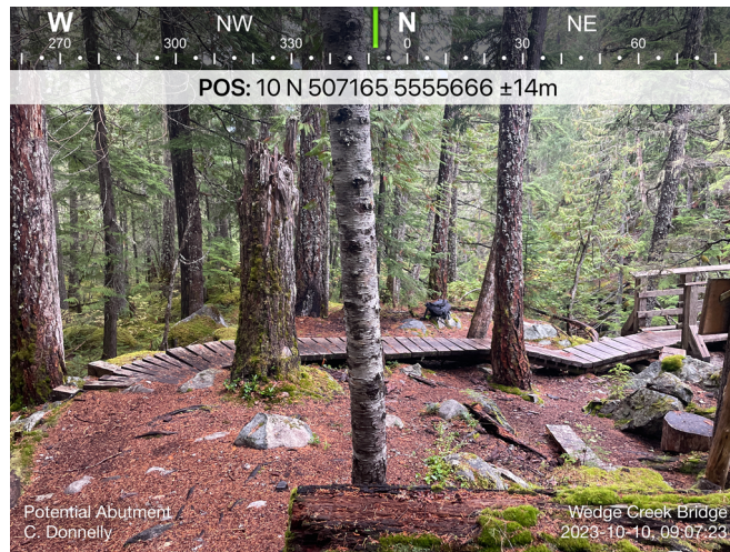
Figure 2: Southwest side of the existing bridge – woodwork leading to the existing bridge.
