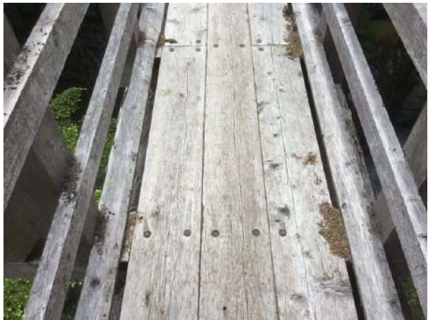
Photo 6 Typical deck condition
