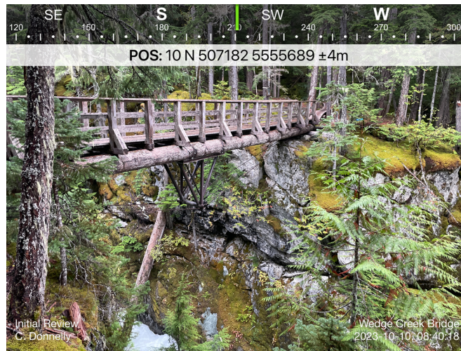
Figure 4: Exposed bedrock beneath the southwest bridge abutment.
